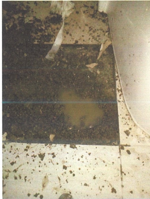
Figure 3.3.4 : Water coming out from floor.
