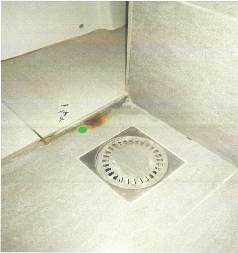
Figure 3.4.1: An opening gap or grouting between tiles.
