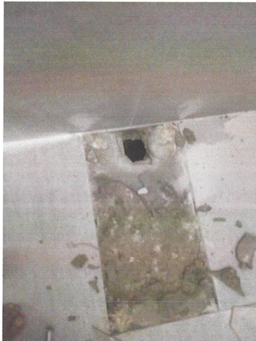
Figure 3.4.5 : Big hole on slab covered by tile.
