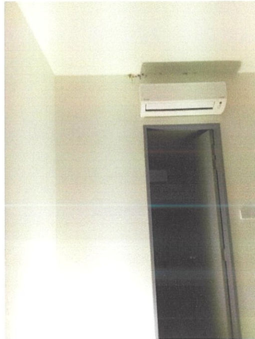
Figure 3.2.1 : Water mark on the top of air-conditioner.
