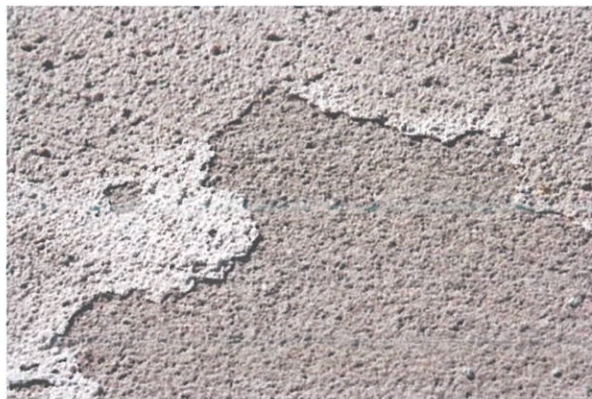
Figure 3.3.2.1: Blisters on slab
