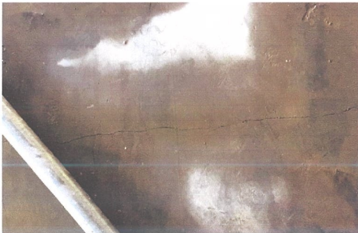
Figure 3.3.1.1: Example of cracking
