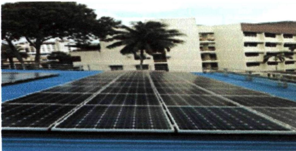
Fig. 3 Example of a 10 kWp GC system installed at GERC, UiTM Shah Alam, Selangor Darul Ehsan, Malaysia.
