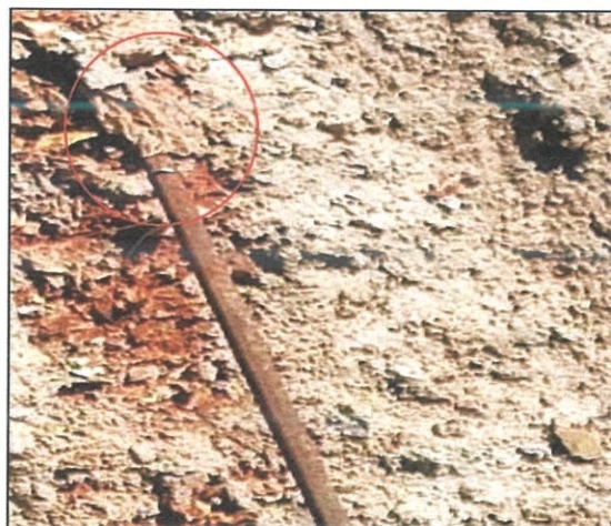
picture 3.8: actual distance of slab
