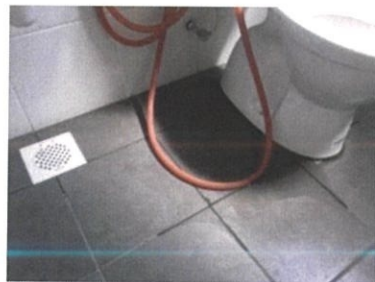
Figure 24 : Stagnant in toilet
