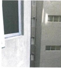
Figure 21 : Hairline crack outside the unit
