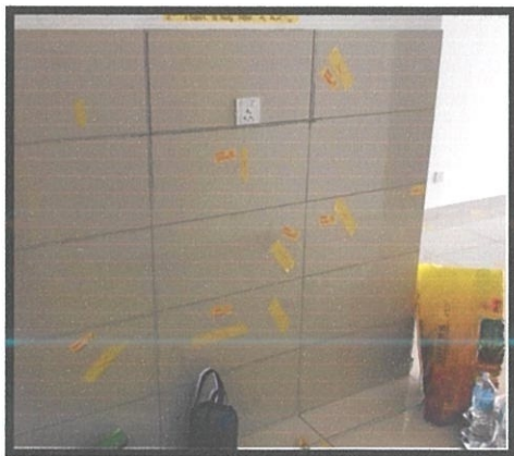
Figure 3.2 The owner put stickers on the tiles are hollow
