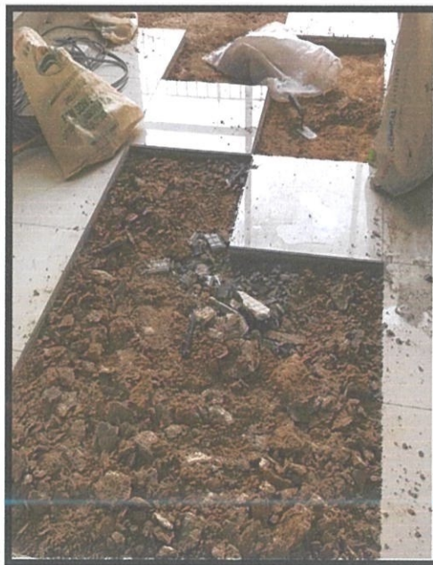
Figure 3.5 Deficiency of screeding
