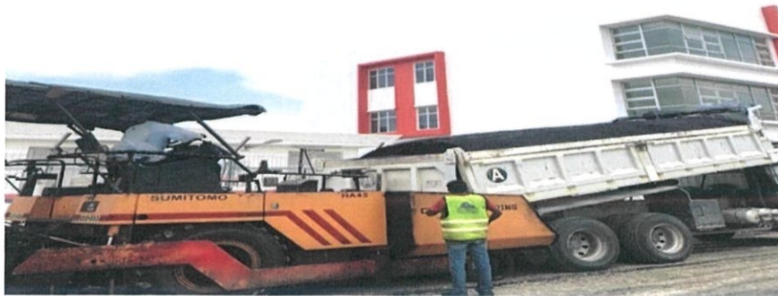
Figure 2.8 – Shows the lorry loading the concrete paver with Asphaltic Concrete Binder Course, ACBC 20
