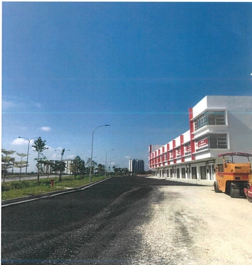
Figure 2.4 – Shows half of the base road has been coated with prime coat (SS1K)
