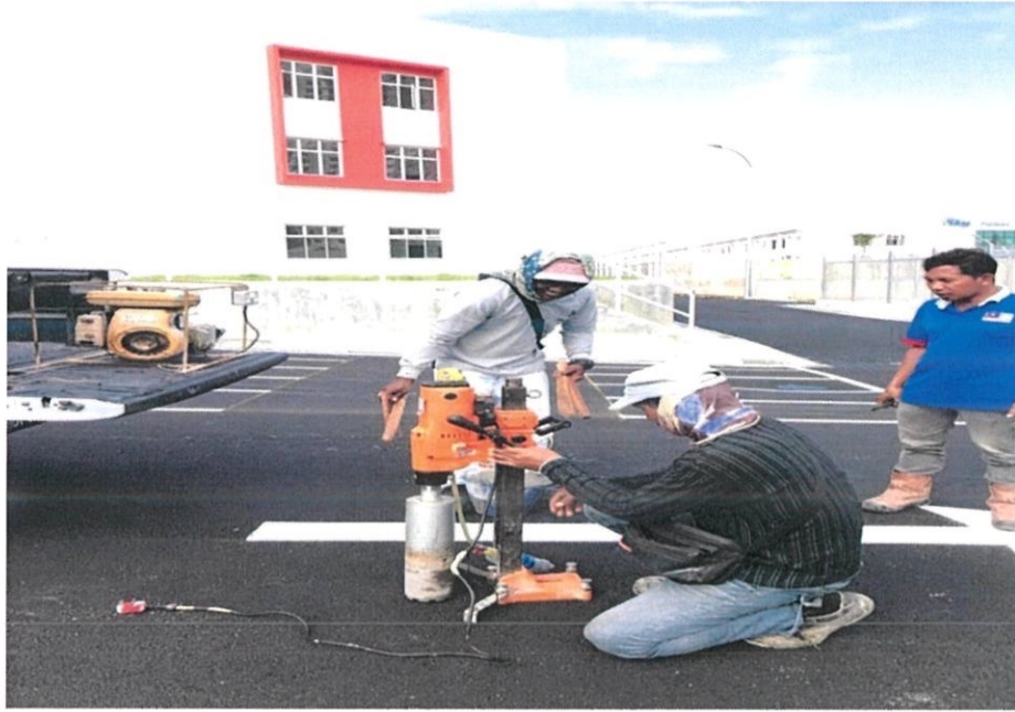
Figure 2.13 – Shows the core drilling machine that being used to extract the coring sample
