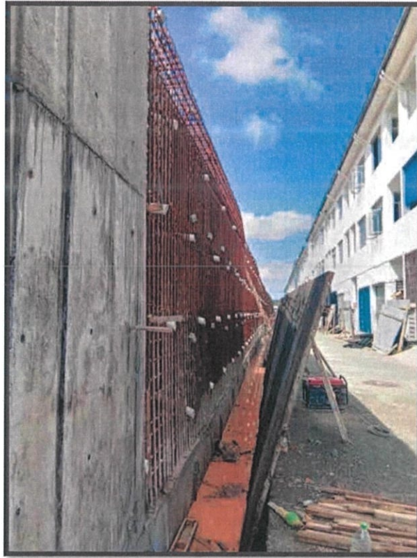
Figure 42: The steel formwork shifted adjacent part of retaining wall.
