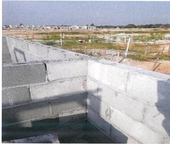
Figure 3.24: Reinforcement not available
