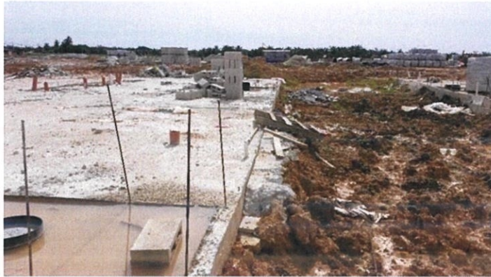
Figure 3.23: Floor is Not in Good Condition
