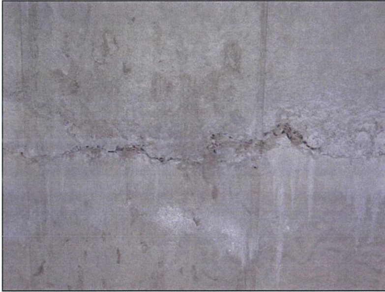
Figure 3.13 Cold joint on a wall
