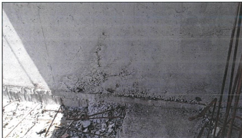
Figure 3.12 Concrete segregation on a wall
