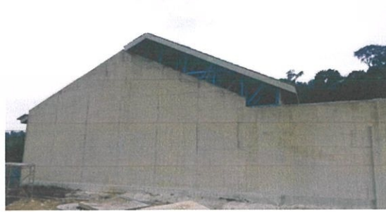
Photo 3.14: The wrong location of roof truss
