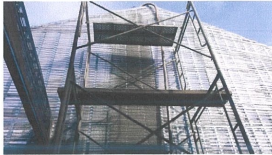
Photo 3.12: The mortar was filled into the wall panel using the mortar pump
