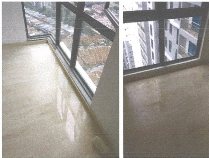
Figure 3.34: The timber board soaked in water
