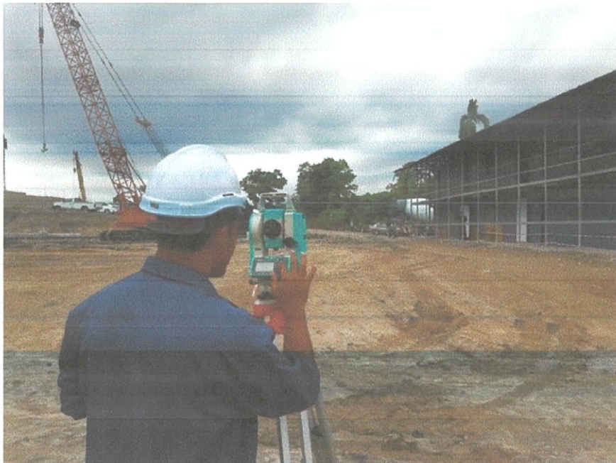
Figure 3.10 Surveyor conducted setting out of pile location for Main Block of Cardiology Block, Hospital Serdang.
