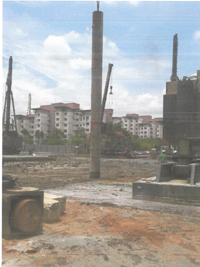
Figure 3.17 The jacked-in machine lifted 'dolly' into the grip to conduct set criteria.
