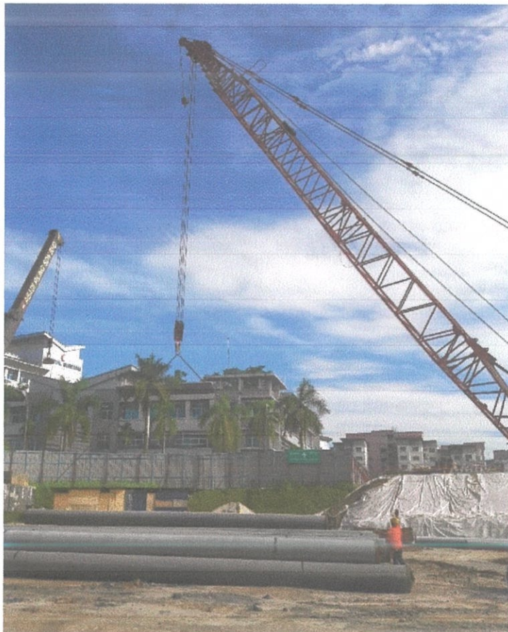
Figure 3.14 Spun piles are placed from another location to near pile location to ease the process.
