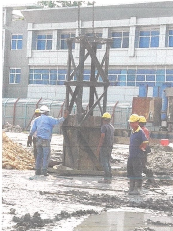
Figure 3.22 The cage of hammer was lifted by crawler crane from one place to tested pile location.
