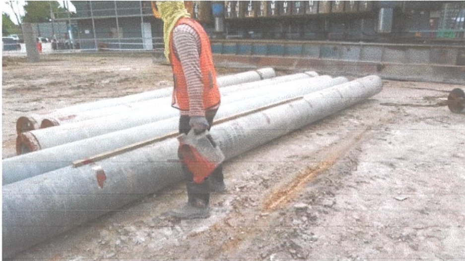
Figure 3.12 Worker measuring and paint spun pile size 600mm with 1m each along the pile with red paint.
