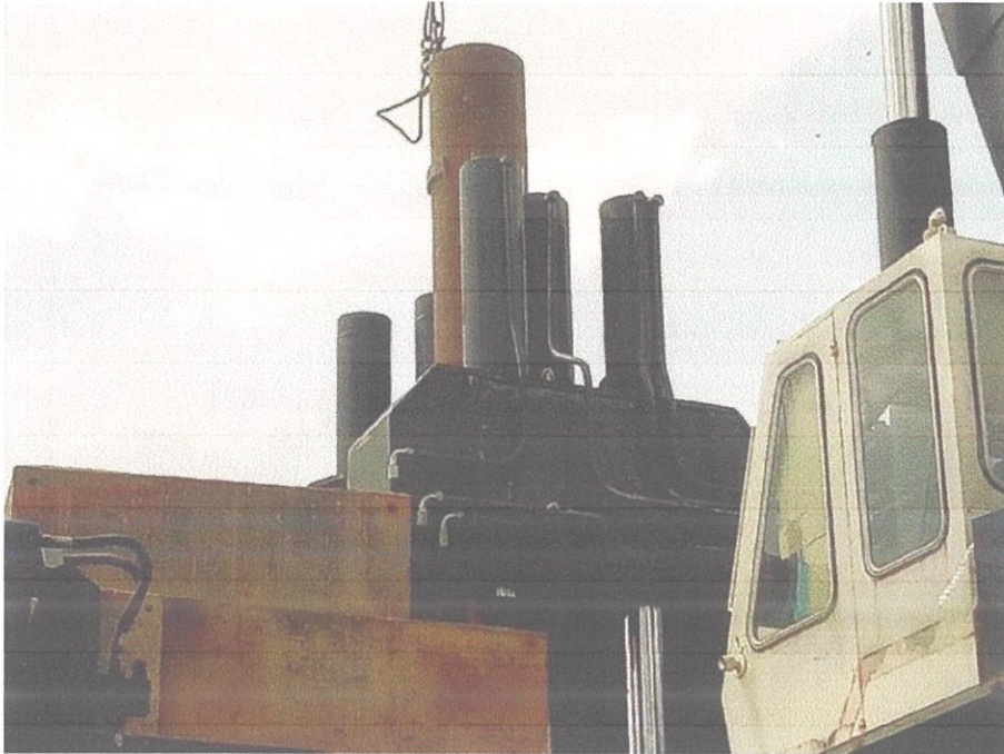
Figure 3.15 The installation of 600mm diameter spun pile into jacked-in machine 10 using 6 cylinder.
