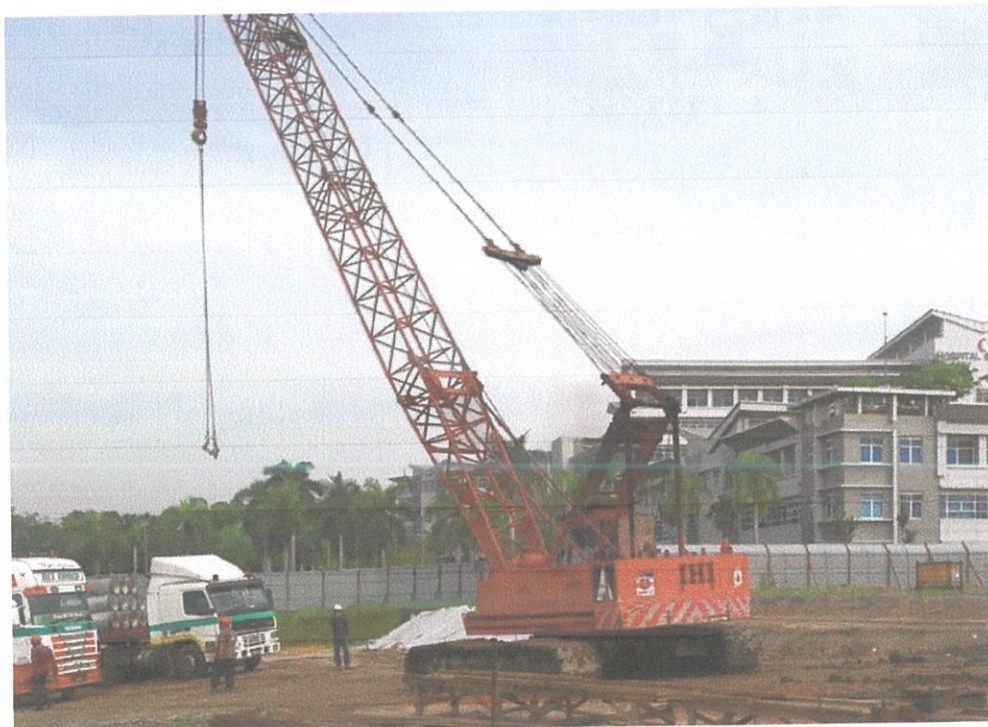
Figure 3.9 Crawler crane use to lift spun pile from the trailer truck delivered on site.
