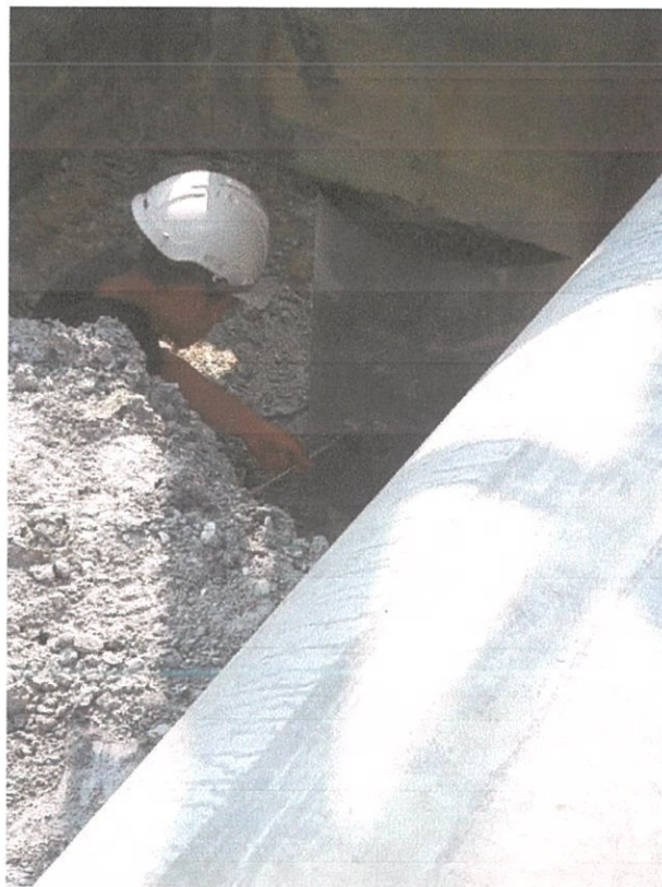
Figure 3.26 appropriate sizes of holes were drilled on the surface of tested pile of sensitivity sensor and connected to pile driving analyser.
