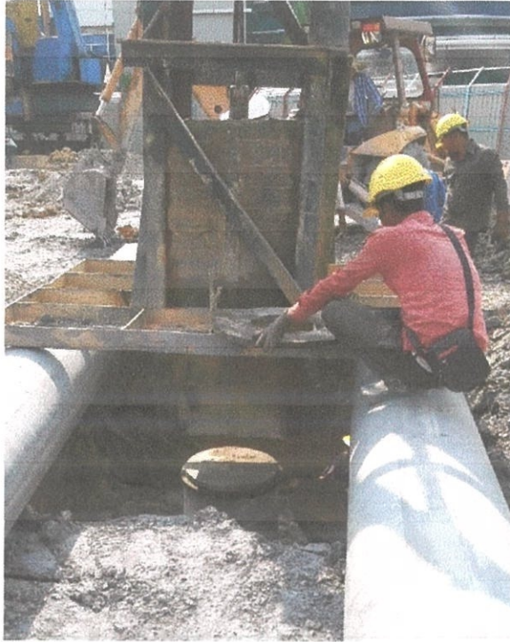
Figure 3.23 Hammer drop was placed on tested pile and ready to be tested.
