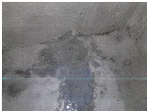
Figure 3.32: Watermarks on slabs
