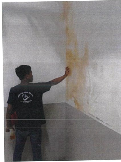
Figure 3.26: Water leaks on wall
