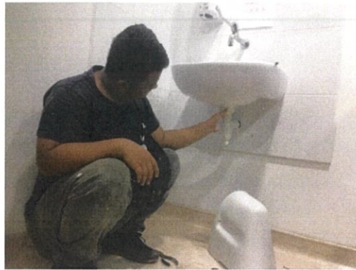
Figure 3.23: Worker wrapped putty around the leak area
