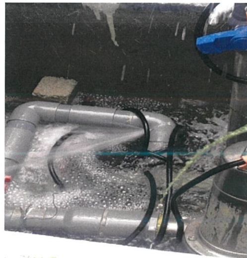
Figure 3.7: Water leaking from pipe
