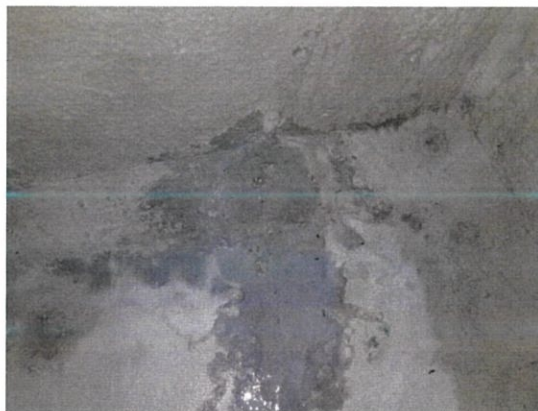
Figure 3.25: Water leaking on slabs
