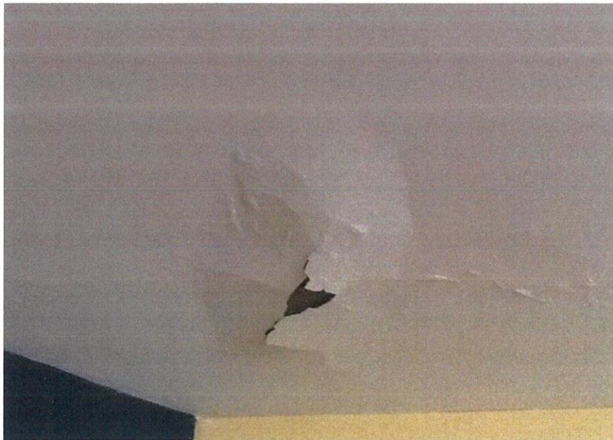
Figure 3.9: Plaster ceiling cracks
