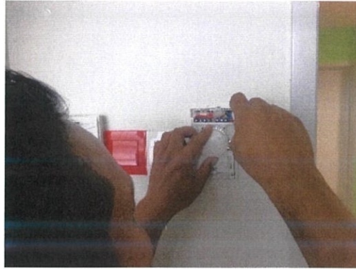
Figure 3.8: Thermostat wire trip
