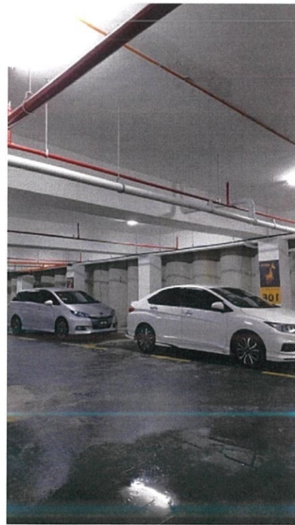
Figure 3.5: Water leaking from ceiling
