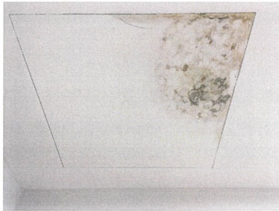
Figure 3.17: Fungus on ceiling plaster
