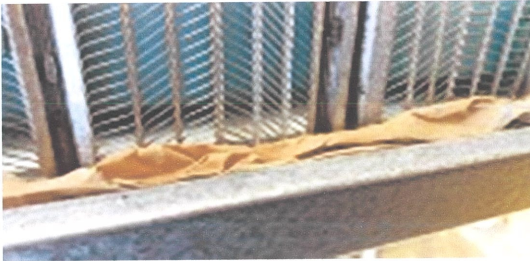
Photo 3.24: Gap between netting
