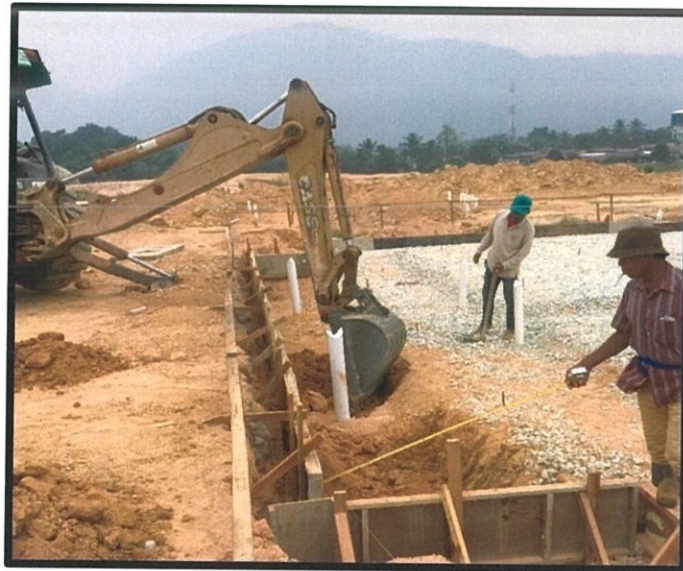
Figure 3.33 There is no safety equipment
