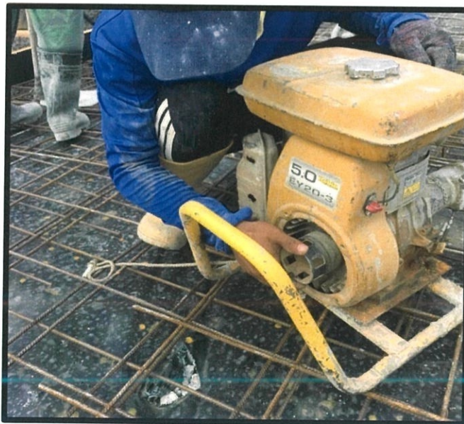
Figure 3.35 The vibrator starter already broke
