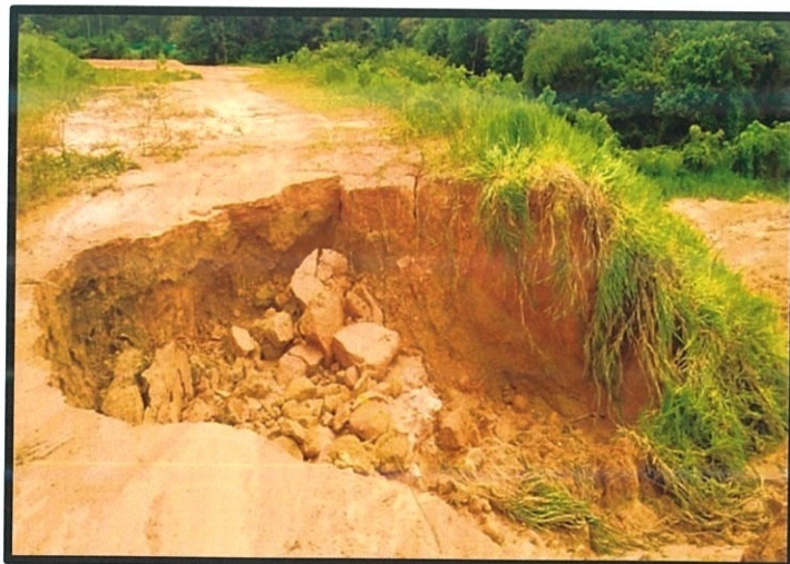
Figure 3.32 The temporary road eroded
