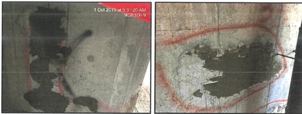
Figure 14: Example honeycomb that have been complete patching
