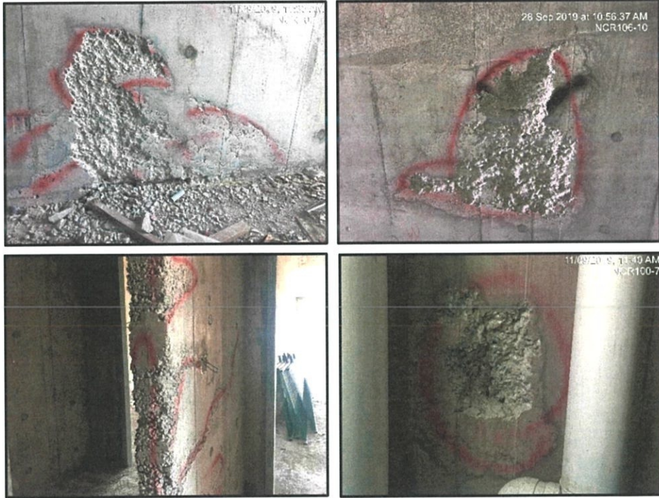
Figure 7: Example of minor defective honeycomb
