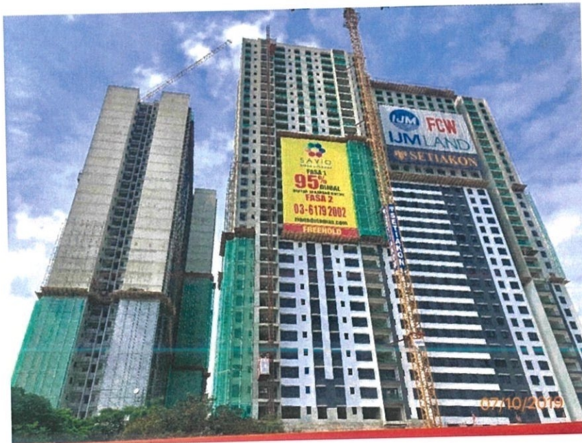
Figure 3: View of the progress building the left is Tower A, then Tower B.
