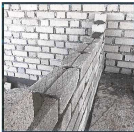
Figure 3.12 Excess mortar that was embedded into the cement mortar.
