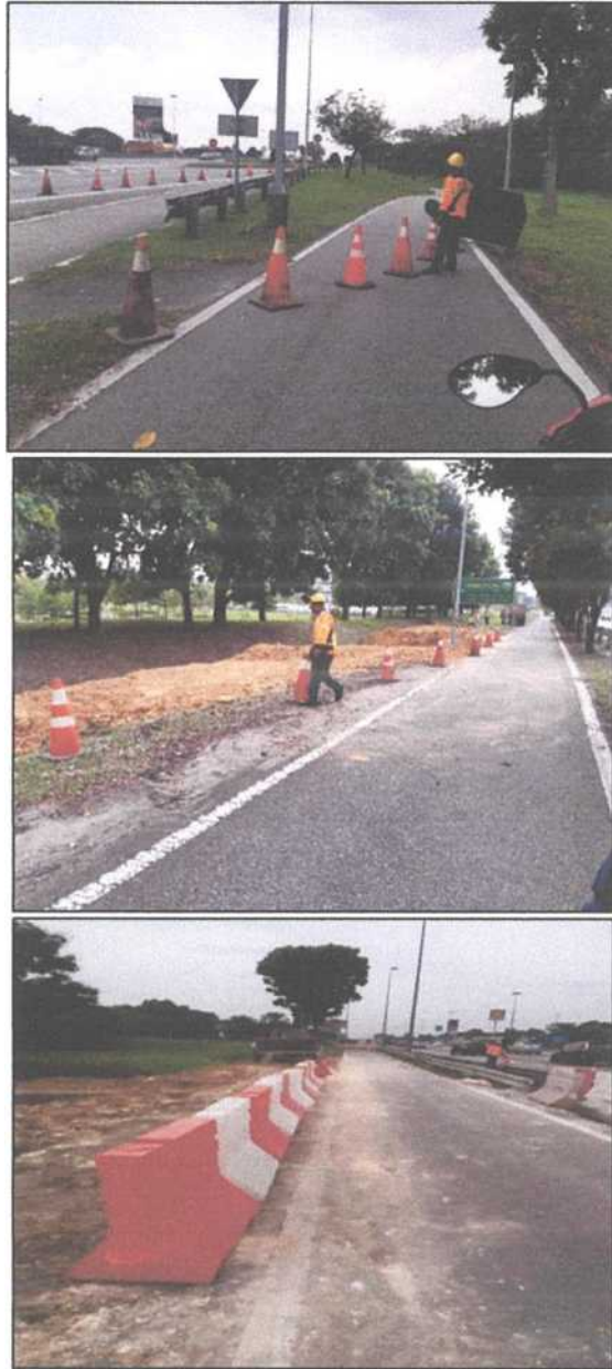
Figure 13.0: Traffic Management System (Courtesy FE Sdn Bhd)
