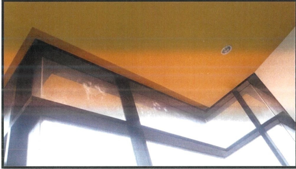
Figure 3.13 : Dirty glass window at Level 7 of MKH Boulevard
