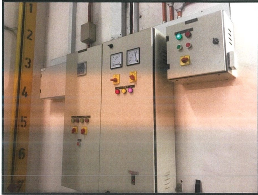
Figure 3.9 : Electric switchgear at HT Switch Room 1, MKH Boulevard
