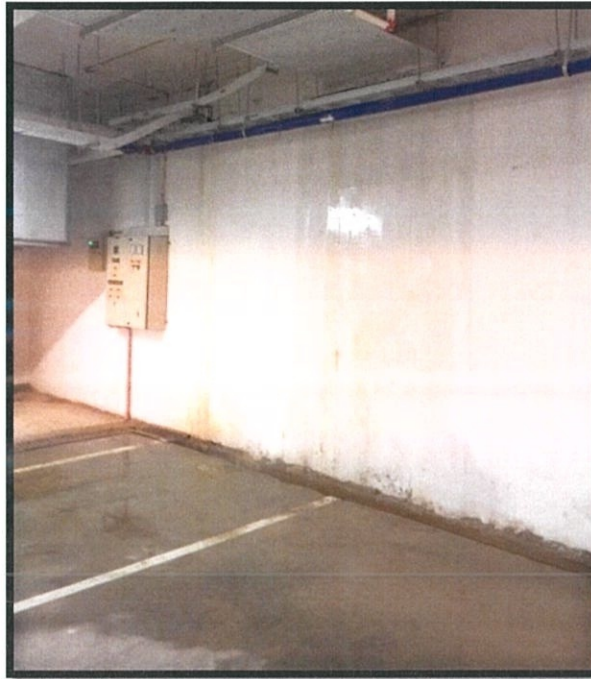
Figure 3.14 : Water leakage into basement
