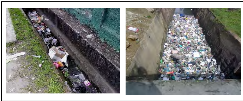
Figure 2: Example of Water Contamination
