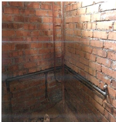
Figure 6.4 The Upvc concealed pipe installation
