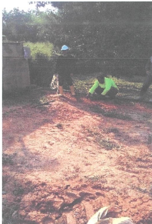
Figure 3.2 indicates two workers had done setting out by marking using sledge hammer.
