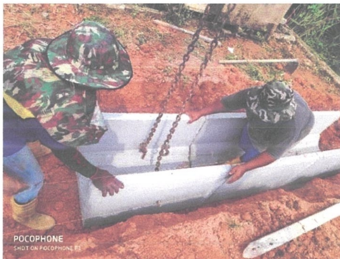
Figure 3.7 show the installation of the precast U-drainage in sizes 750mm x 750mm.
