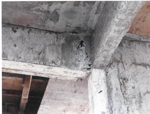
Figure 3.26: Honeycomb at first floor beam.
