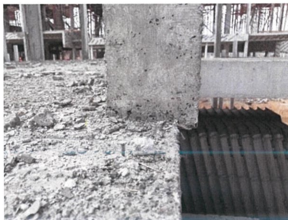
Figure 3.27: Inaccurate dimension or placing of column at first floor.
