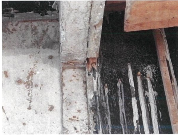
Figure 3.28: Left over formwork which got stuck in the concrete due to inaccurate installation of formwork.
