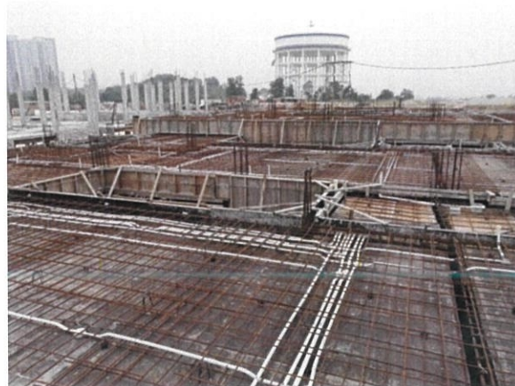
Figure 3.11: Usage of tips coated metal chairs and circular spacers as concrete cover.
