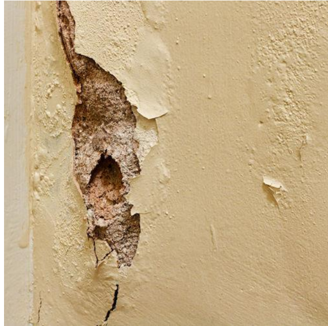
Figure 3.4.3 above shows delamination crack.
