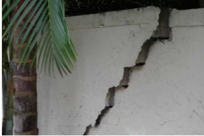
Figure 3.4.2 above shows settlement crack.
