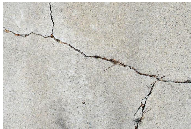
Figure 3.4.1 above shows hairline crack.
