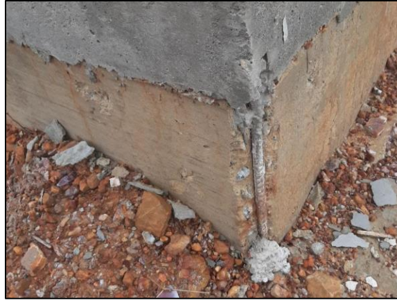
Figure 3.20: Eroded Concrete of Ground Beam.
