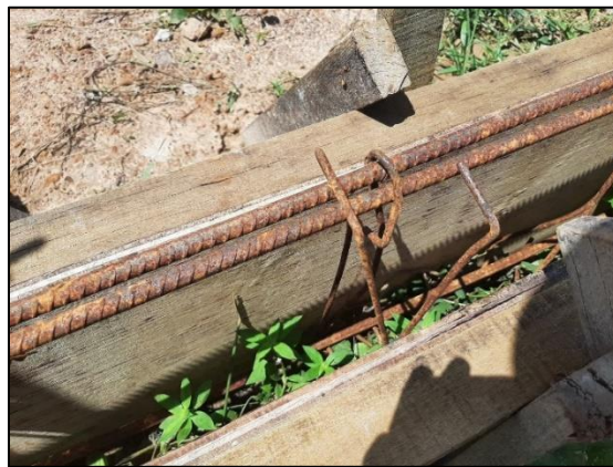
Figure 3.18: The Reinforcement Link Was Not Tied Properly.
