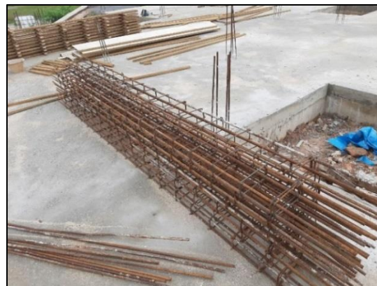
Figure 3.12: Y12 Steel Bar That Has Been Fastened Together with R6 Steel Reinforcing Link.
