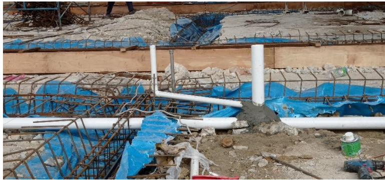
Figure 3.2.6 (Steel pipe and PVC pipe are used for the internal cold water plumbing)
