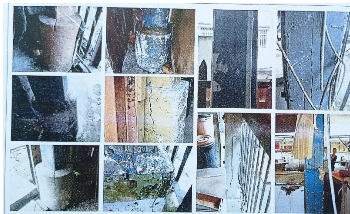
Figure 3.2.1 (example of wood damaged and concrete pole damaged)
