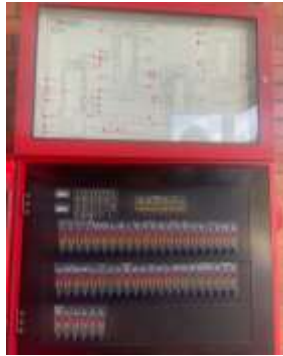
Figure 3.2: Main fire alarm control panel
