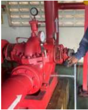
Figure 3.28: jockey pump system
