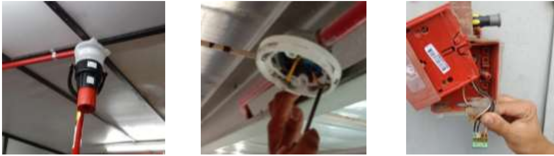
Figure 3.24: inspection and maintenance of Fire Alarm Systems.
