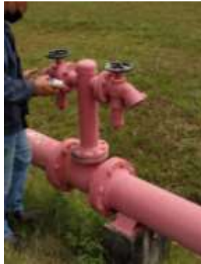
Figure 3.8: External fire hydrant
