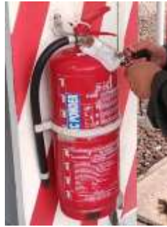
Figure 3.6: Portable fire extinguisher.
