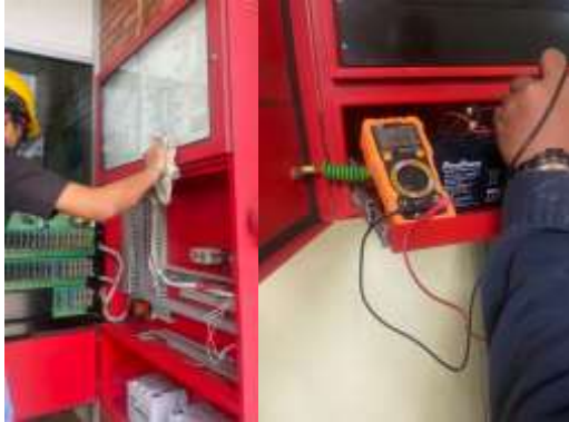
Figure 3.23: inspection and test of Main Fire Alarm Panel
