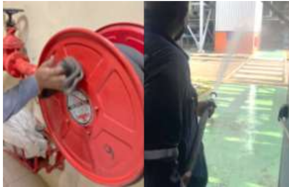
Figure 3.26: testing the hose reel
