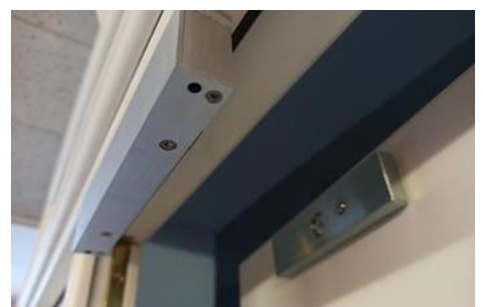
Figure 3. 32: Installation of Door Contact and EM Lock at the site (close view)
