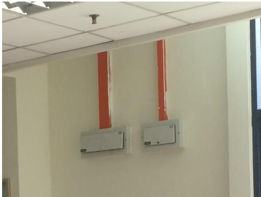
Figure 3.4.7 Paint stains on wire casing
