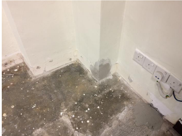
Figure 3.4.3 Cracks in walls that have been filled with cement mixture
