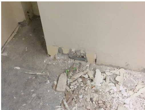
Figure 3.4.1 Damaged wall paint
