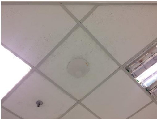
Figure 3.4.4 Messy paint on ceiling with minor stain on its steel frame
