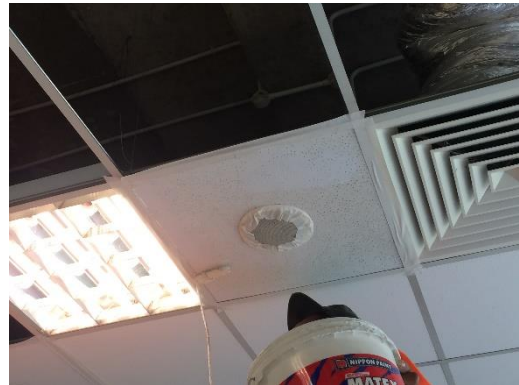
Figure 3.4.5 Device on ceiling that has been covered with masking tapes
