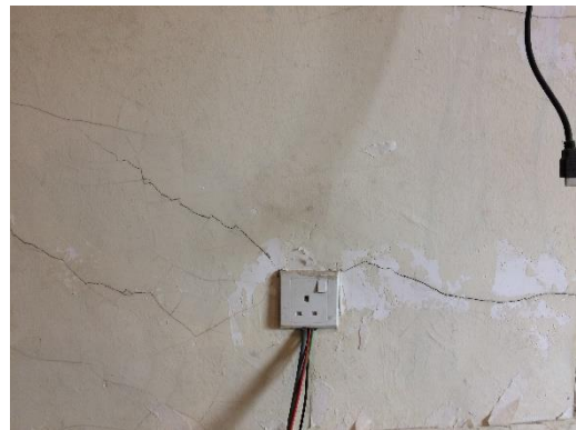
Figure 3.4.2 Crack lines on the wall
