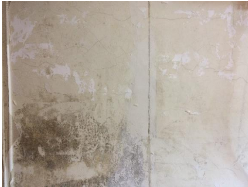
Figure 3.4.12 The dark and moldy stains on wall
