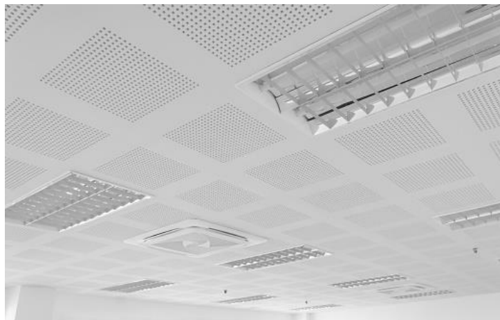
Figure 3. 15: Example acoustic ceiling
