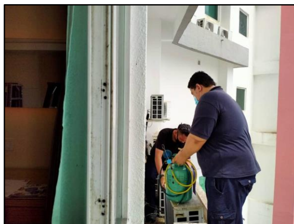
Figure 26: Gas Top up Process
