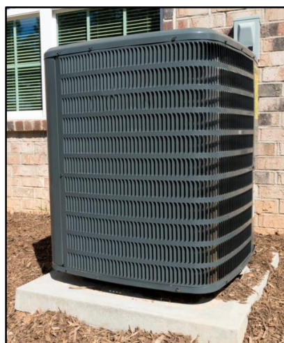
Figure 9: Aircond Condenser Coil
