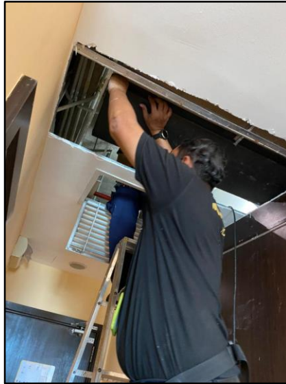
Figure 20: Taking Out the Motor Blower Fan Process
