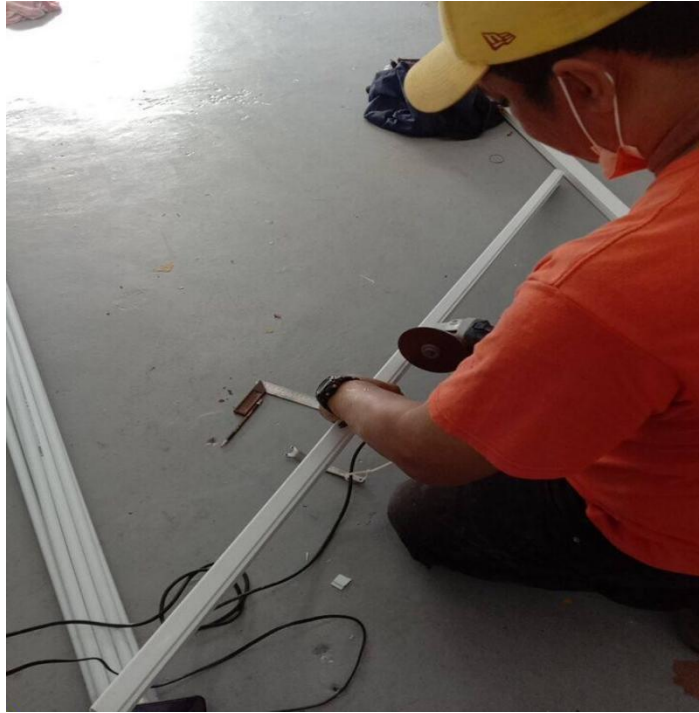
Photo 3.2: Cut casing cover for wiring
