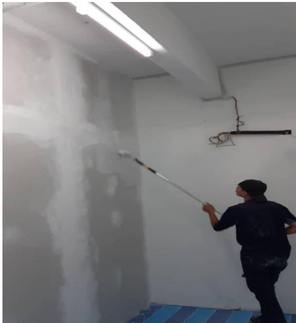
Photo 3.7: Paint Plaster Area
