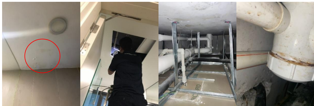
Figure 3.2.4d, e, f & g: Inspection of leaking
