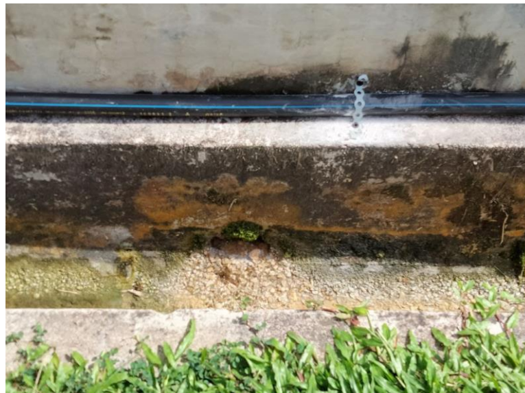
Figure 3.3: Water comes out slowly as there was a blockage in pipe.
