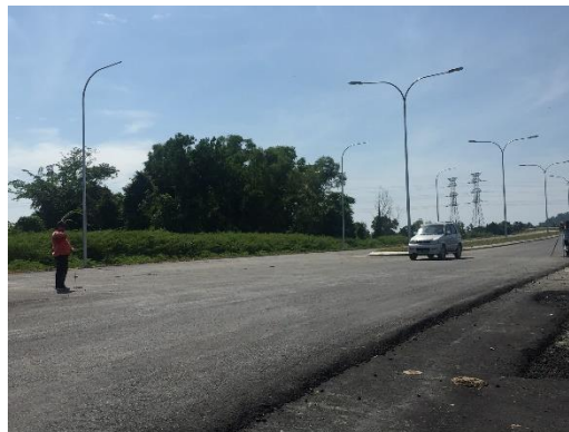
Figure 3.21: Street lighting installation at the highway.
