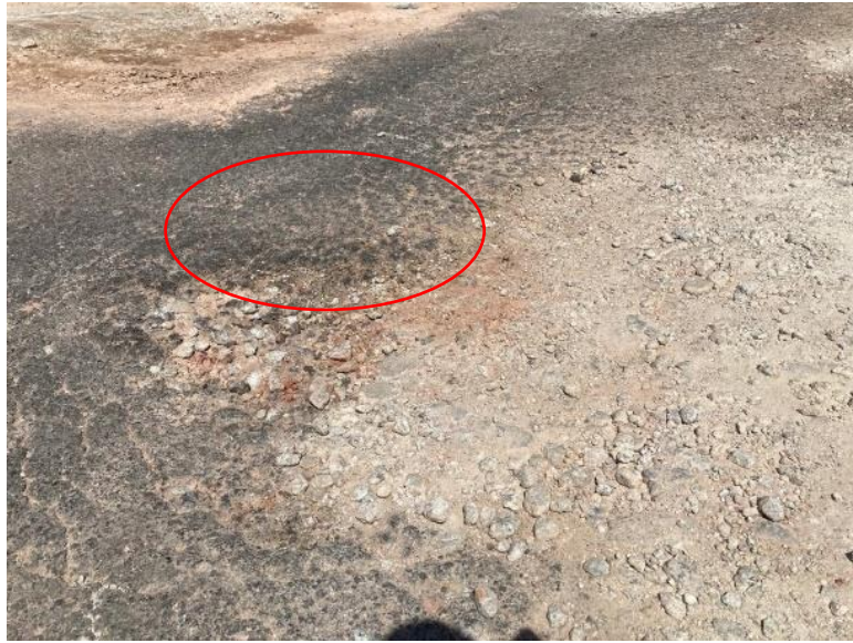
Figure 3.8: Potholes on the road surface
