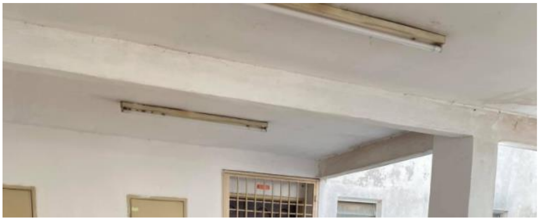
Figure 3.30: The Corridor Fluorescent Lamps
