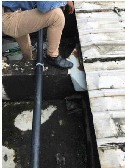
Figure 4.1: The Condition Gutter at Roof Top
