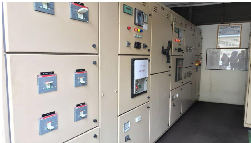
Figure 3.28: The Main Switch Board
