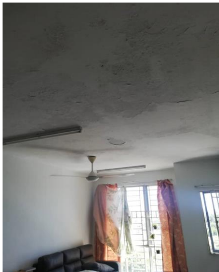
Figure 3.31: Peeling off paint on the ceiling
