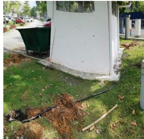
Figure 3.45: Condition before refill soil work back after the leaking pipe has been rectify
