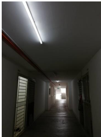
Figure 3.50: Condition of broken LED lamp
