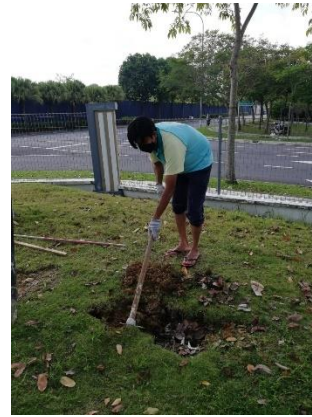
Figure 3.43: Dig soil to find the leaking pipe
