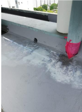
Figure 3.36: The condition of the waterproofing that not fully dry
