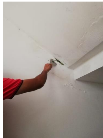
Figure 3.47: Remove mould growth from the area
