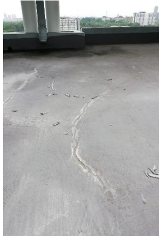
Figure 3.33: Hacking affected area of old waterproofing
