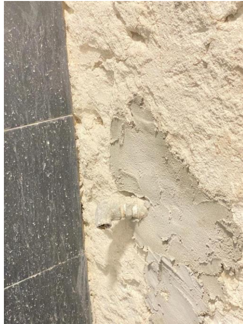
Figure 23 water supply pipe
