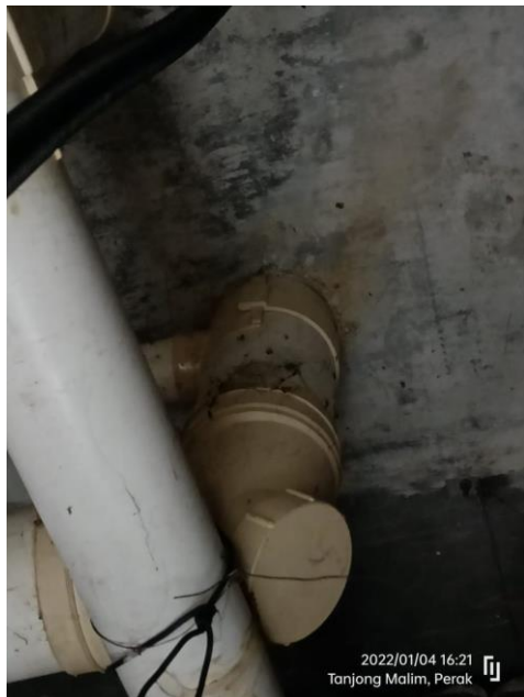
Figure 20 Leaking Inspection on 2nd floor
