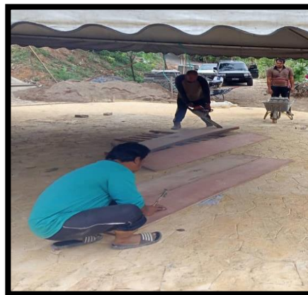
Figure 4.0: Lack of safety site workers
