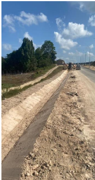
After close up by sand and soil. The surface of the drain will shape to be v shape drain.
