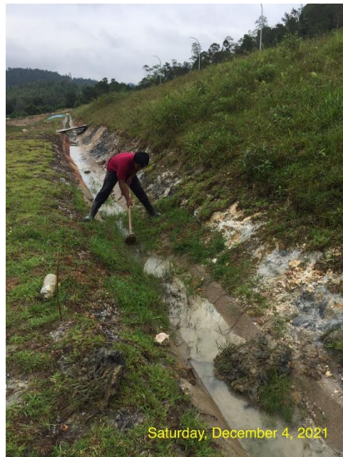
Figure 16: Clogged Drain With Soil
