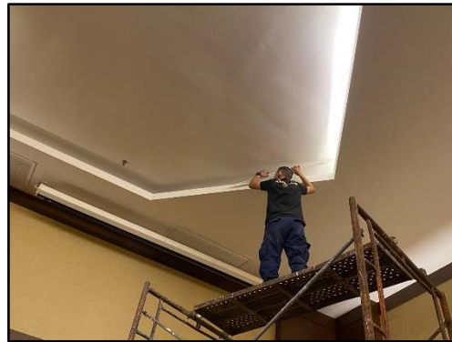
Figure 4.2: The spare part for led lamp was missing at Baba Nyonya Hall.
