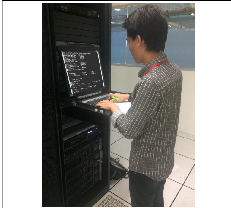
Figure 2.5 Performed Server Preventive Maintenance
