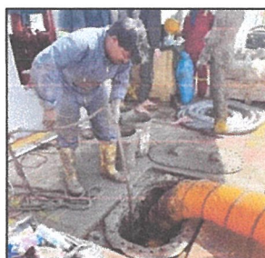
Figure 1: Tank Cleaning Services
