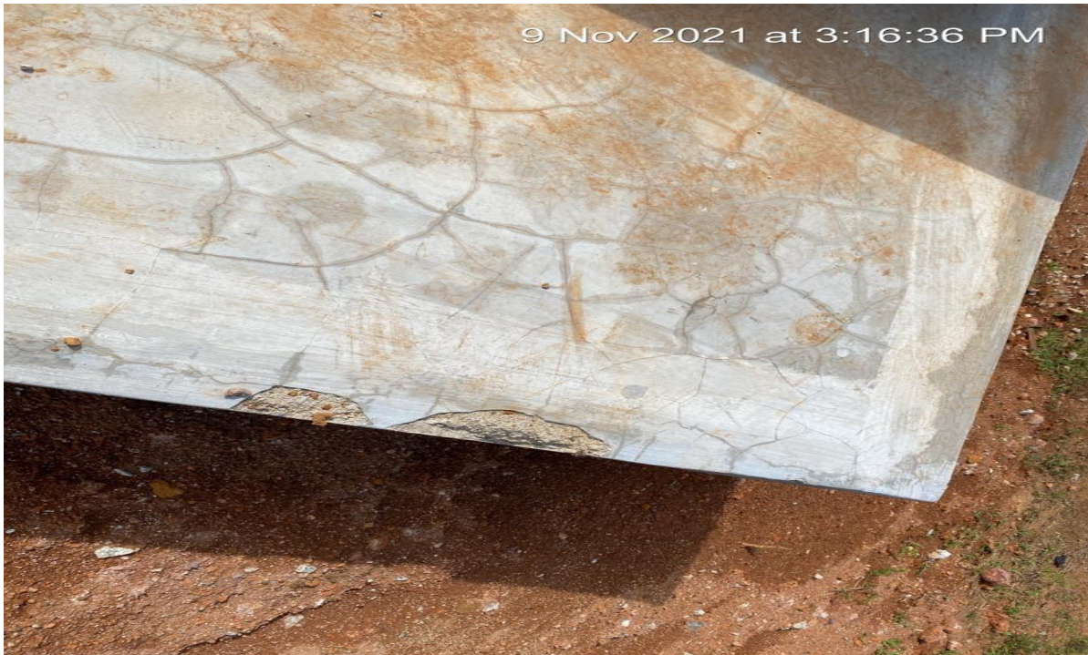
Figure 3.4.1.1 Example of crazing(spiderweb) and cracks at rest pod at site
