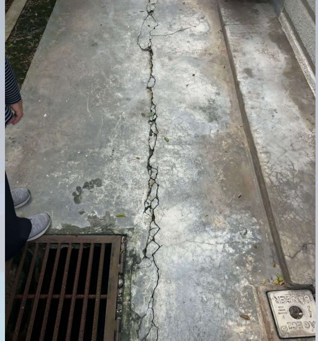
Sample of cracks on the building apron at Kolej Kristal, UiTM CPP.
