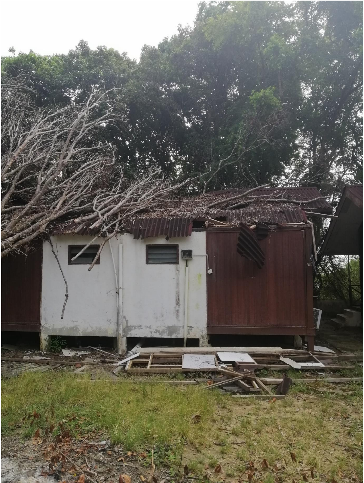
Figure 3.5 Damaged chalet roof because of fallen tree due to storm.
