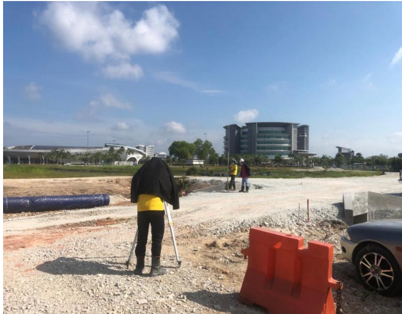
Figure 3.2.4. Checking Premix Level
