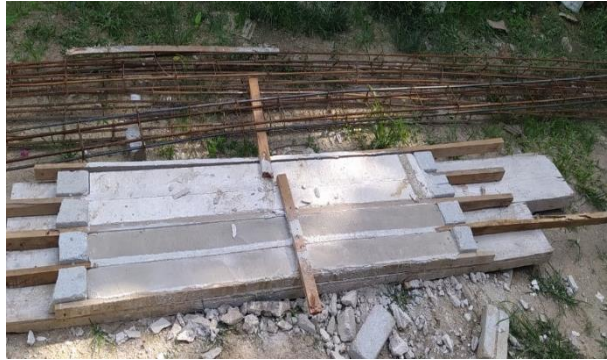
Figure 3.11: the lintel use for load support for opening part of the wall
